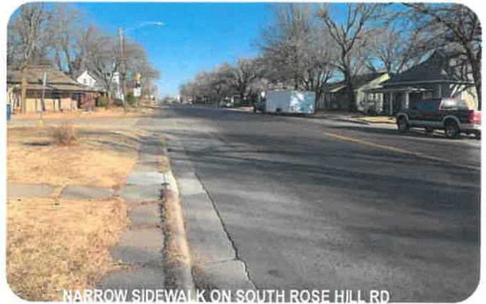
NARROW SIDEWALK ON SOUTH ROSE HILL RD
