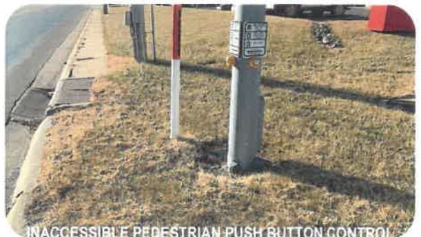
INACCESSIBLE PEDESTRIAN PUSH BUTTON CONTROL
