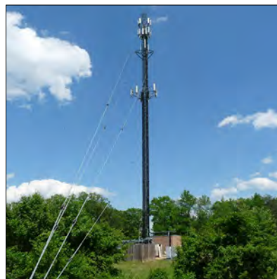
GUYED LATTICE TOWER
