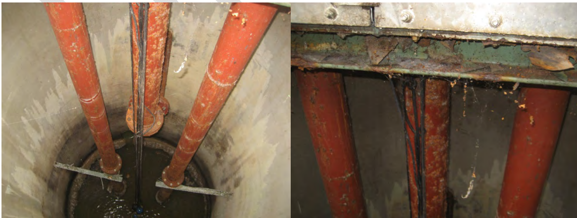
Figure 2 Strode Lift Station Piping and Cover
