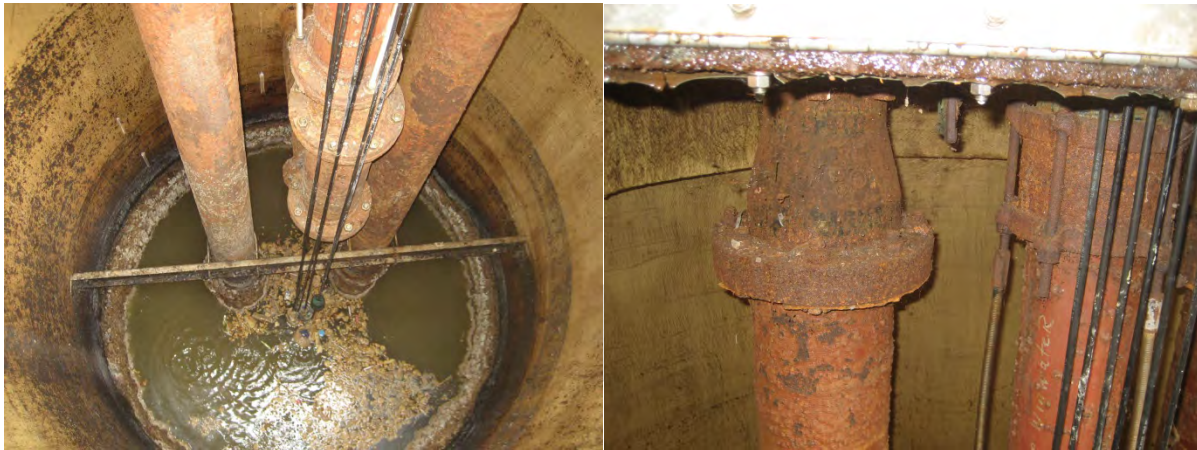
Figure 4 Deer Creek Lift Station Piping
