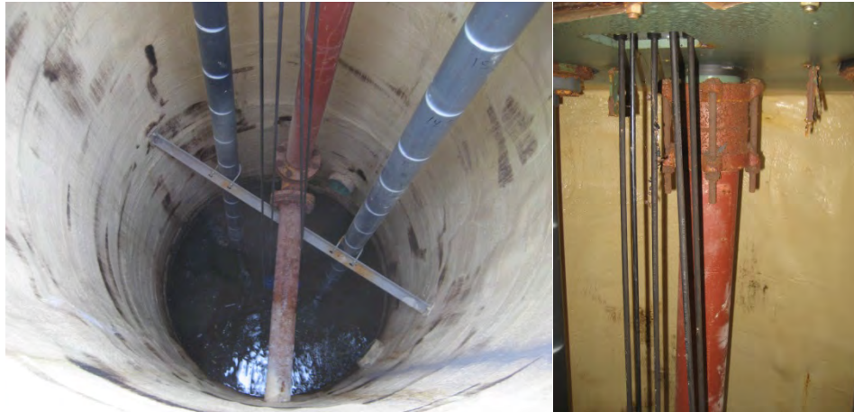
Figure 1 Industrial Park Lift Station Piping and Wet Well
